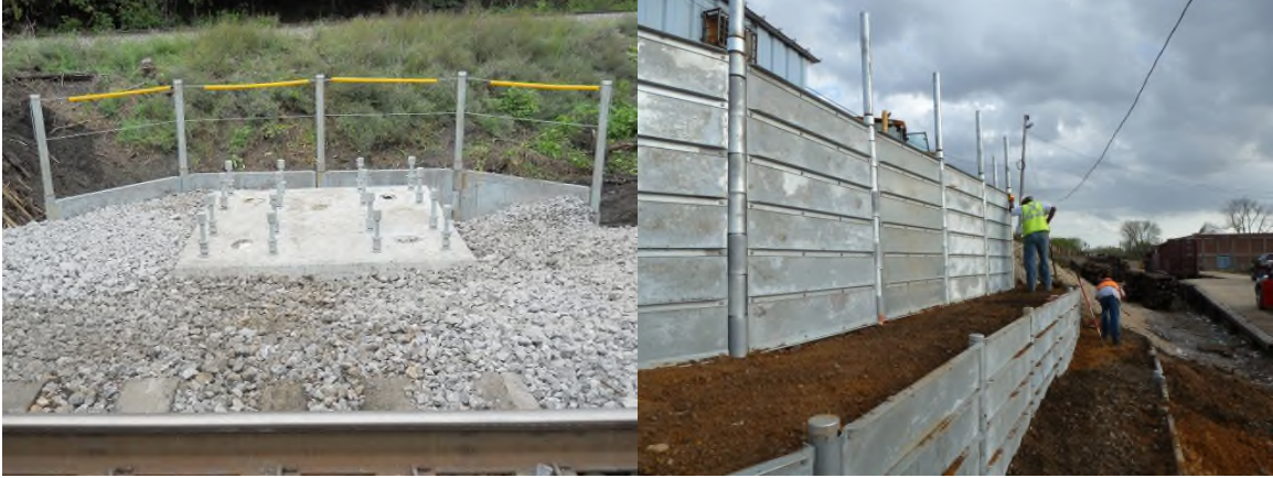
Pipe caps are installed on top of the posts with hex head allen wrench.
